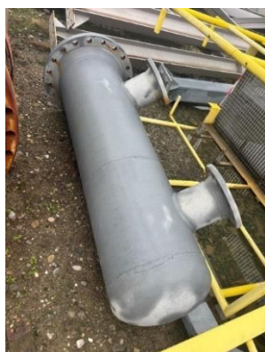
Exchanger under maintenance / repair
