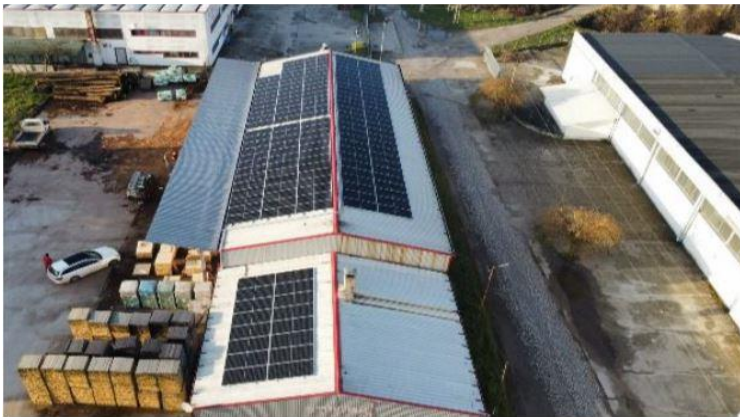
Fig. 2. Placement of the photovoltaic panels on the production hall rooftops.
