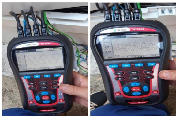
Figure 7. The analyzer located upstream and downstream of the regulator
