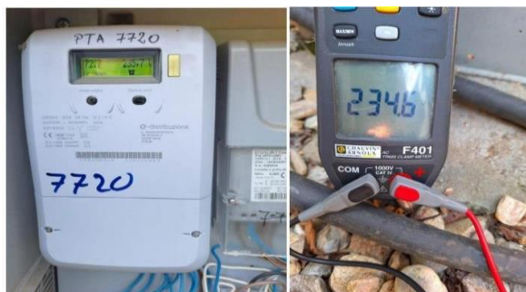
Figure 9. The voltage at the beginning and at the end of the line on which the regulator was placed
