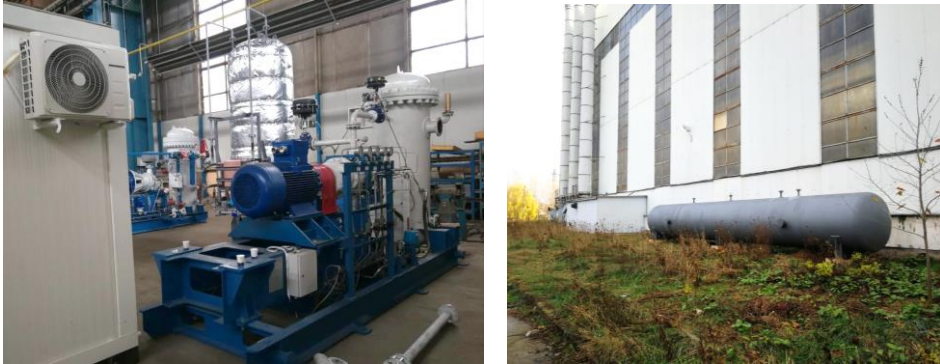
Figure 8. ROCAES plant and air reservoir installed at Popeci, Craiova
