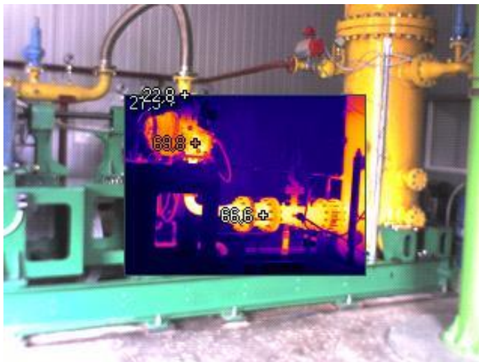
Figure 3. Thermal image compressor.
