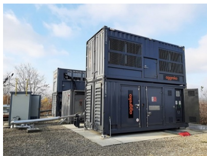
Figure 3. APG power plant with synchronous generators P_i = 1.5 MW each
