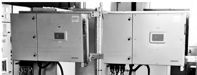
Figure 2 Inverters for A category photovoltaic power plant
