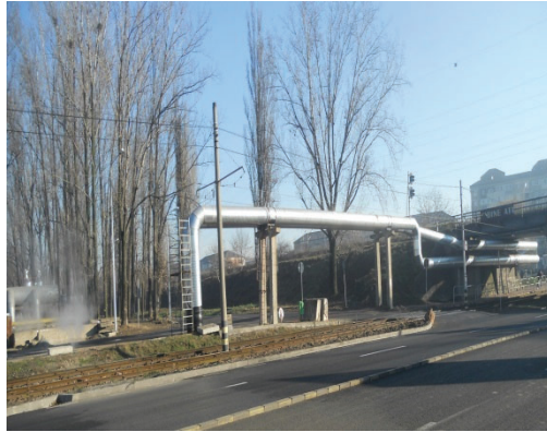
Fig. 20. The primary main pipeline M1 upgraded in 2015 in the area of CFR Bridge from Borsului Road.
